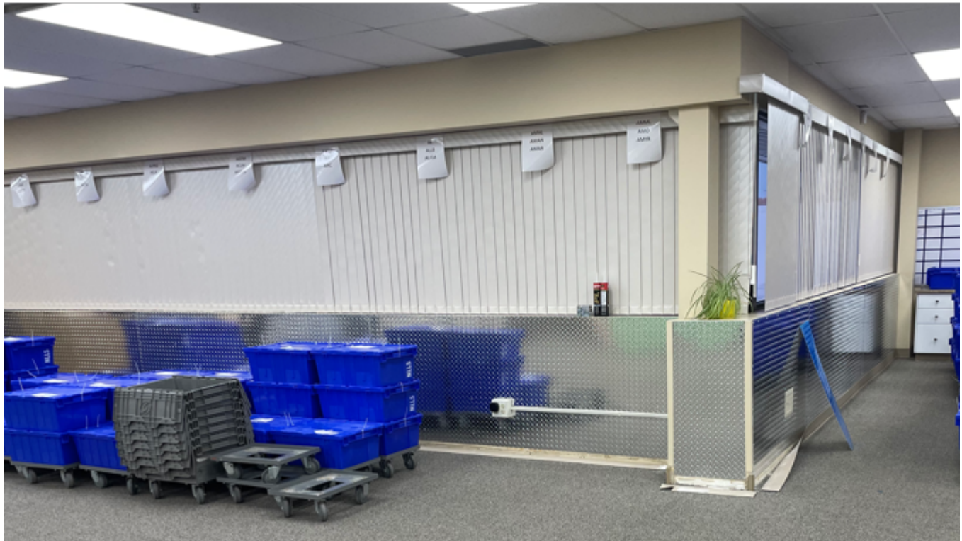
Shiny new metal being installed on the walls in Ops at HQ as part of our regular building maintenance.
